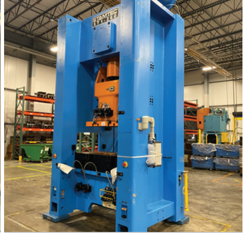
276-Ton Stamping Press installed at Jonesboro
